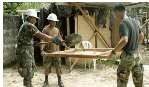
Filipino and U.S. military engineers working at a construction site for a 3 room school building to be added to an existing high school in Sulu, located in the province of Jolo in southwestern Mindanao
